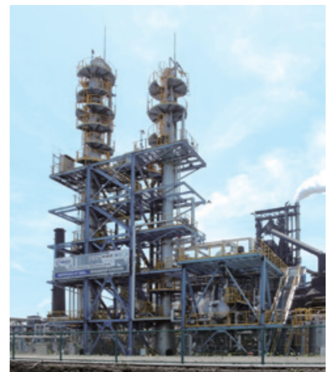
The CO 2 separation and recovery verification plant "CAT-30" in the COURSE50 project
